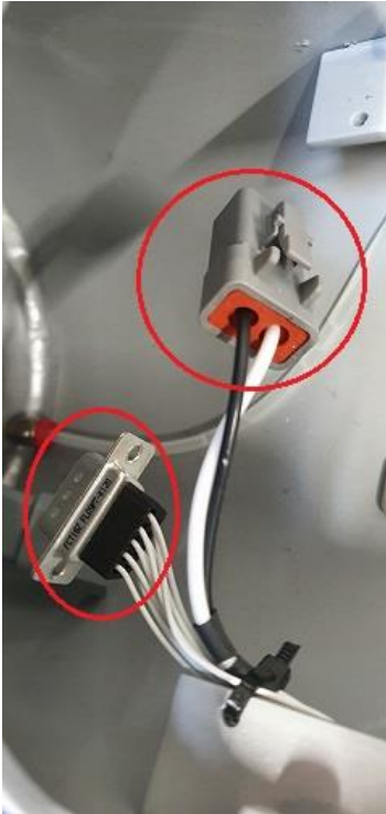
Figure 31 - Power and communication connectors
